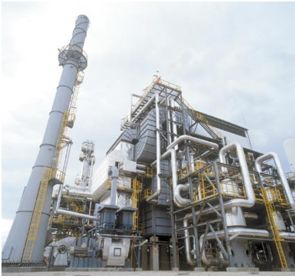
Figure 2. Air Products' hydrogen production facility in Tarragona, Spain.
