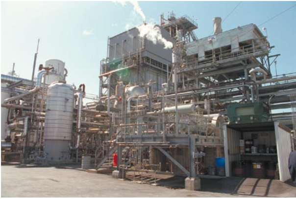
Figure 1. The Martinez 2 hydrogen production facility.
