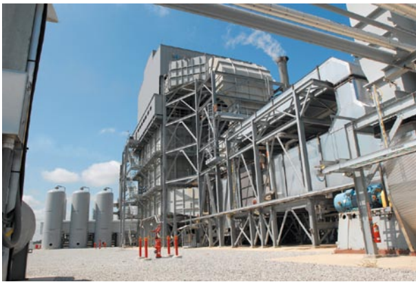
Figure 4. The Sarnia SMR plant in Ontario, Canada.
